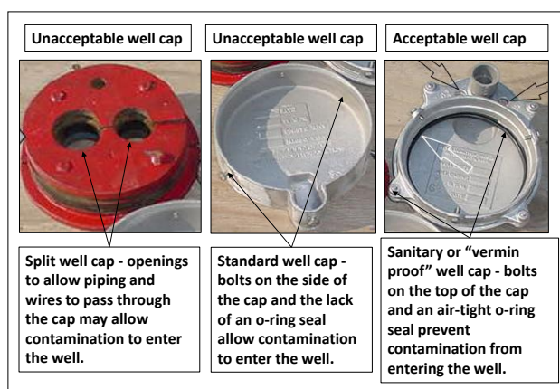
Figure 2: Photos of acceptable and unacceptable well caps
